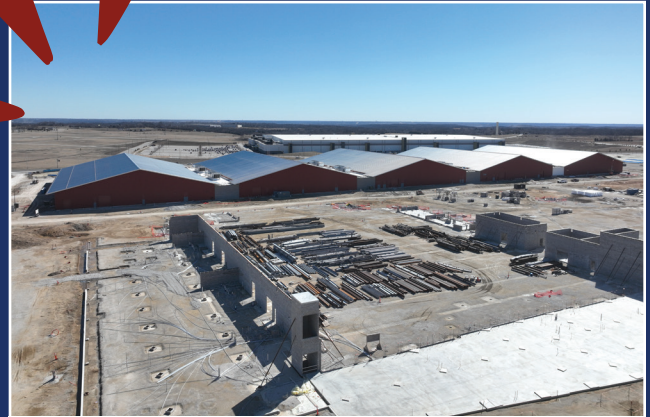
February 2025: Construction progress at the new campus, with the Barns & Exhibition Hall now upright and foundational work underway for the arenas, administrative offices, and the Learning & Engagement Center.
